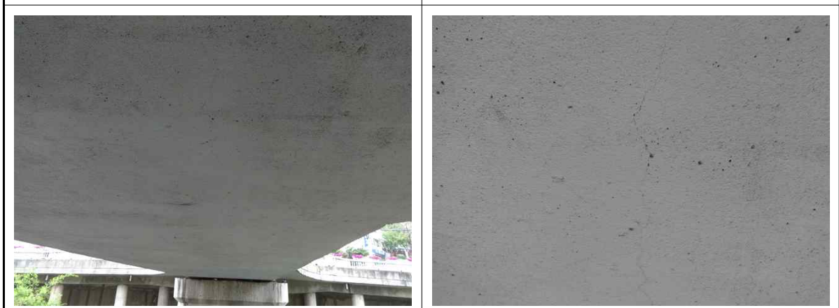
바닥판하면 S1 균열 ( CW=0.1 )
